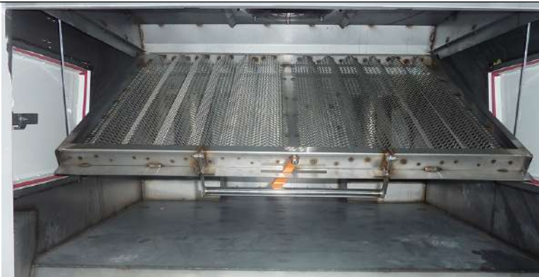
Suction fan screen lowered on its tethers
